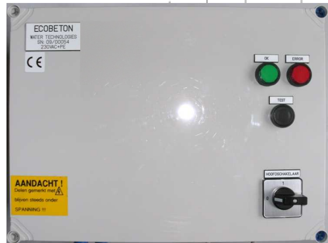
Switch-cupboard, CE conform, cfr. machine-regulations 2006/42/EG.
